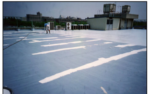
TOPPS SEAL EXCEL is sprayed over POLYPRENE. Next, POLYCORE will be embedded in the wet coating to add extra strength to the roof.
