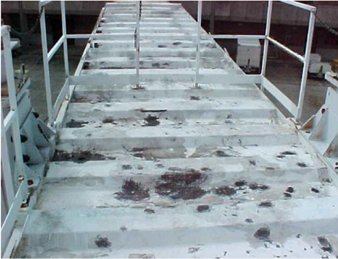
Rust & failure of prior acrylic coating led to decision using waterless Topps Seal™.
